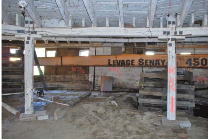
Raising of the round barn to put in place the new foundation
