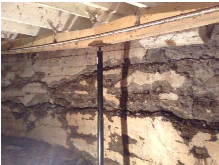
The cracked foundations of the round barn
